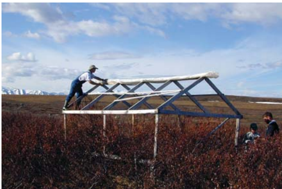
In early June, the covers for the Arctic Long Term Ecological Research (ARC LTER) greenhouse in the tall willow and birch shrub plot are rolled down. The greenhouses are used to increase the summer temperature for several ecosystems in near Toolik Field Station. The covers are rolled up again in mid-August. Credit: Jim Laundre, Arctic LTER
