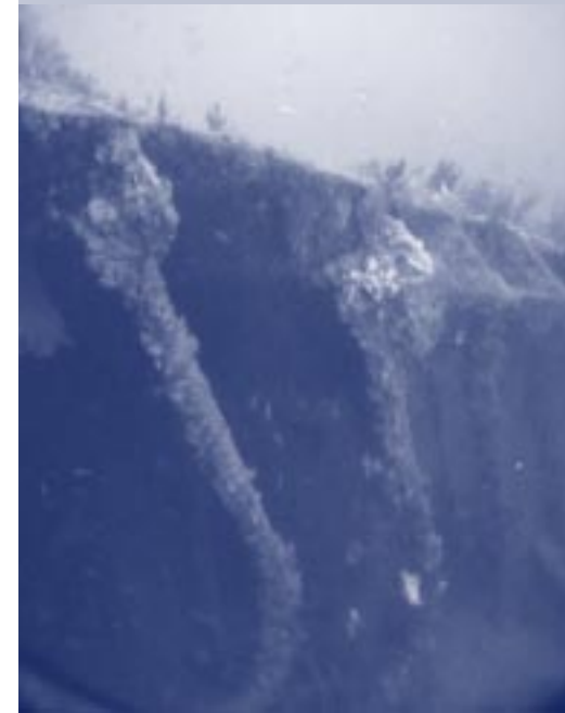
Bent and bowed deck support stanchions and the angled ends of "floor beams" along the port boiler.
