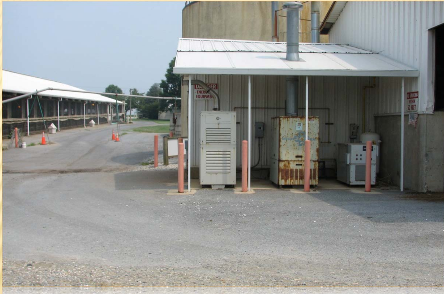
MICROTURBINE AND BIOGAS CONDITIONING
