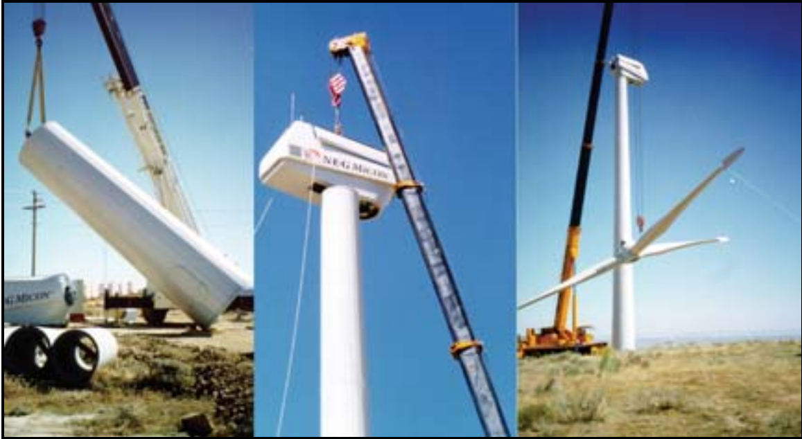
Figure 2-5. Wind Turbine and Crane.
