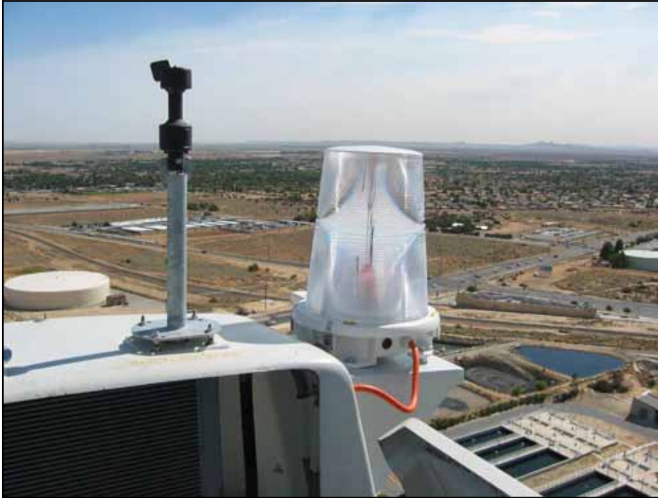
Figure 3-14. Typical Aviation Warning Light.
