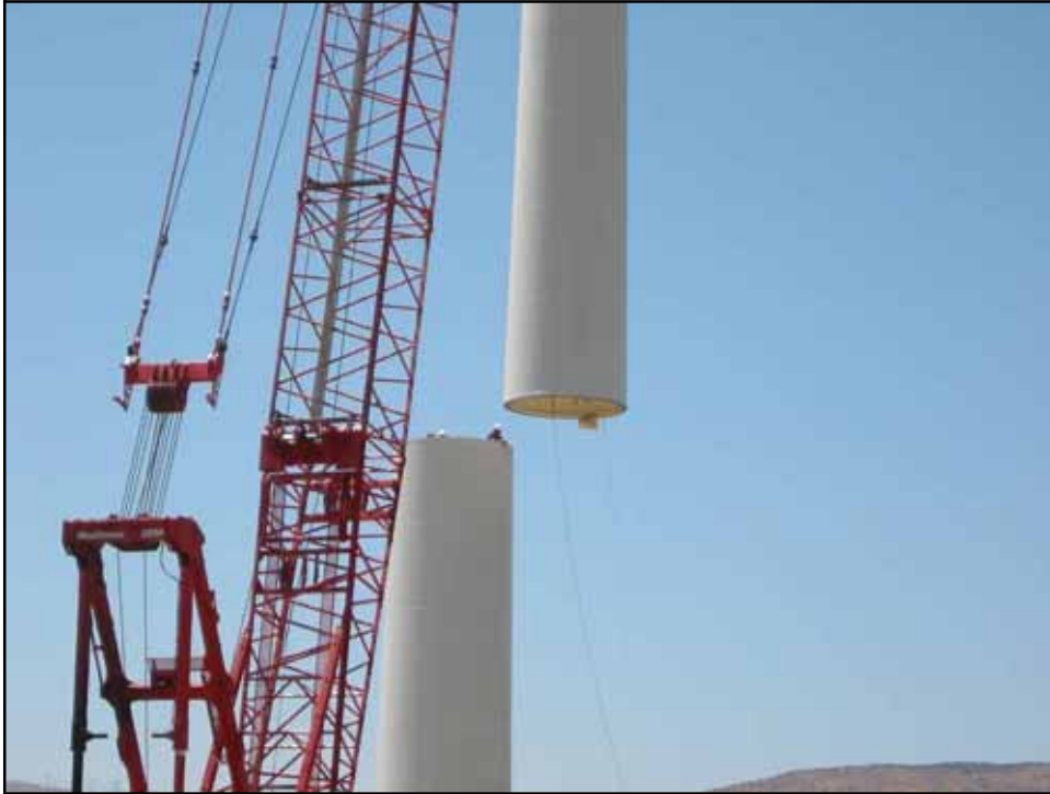
Figure 3-18. Mid-Section Tower Assembly.
