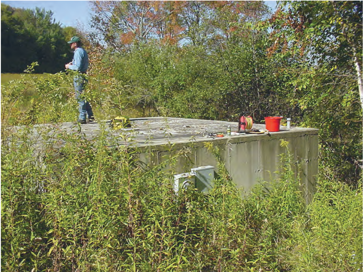
Figure 18. Guilder Hills Spring with combined collection structure, reservoir, and pump house, northward view, Egremont, Massachusetts.
