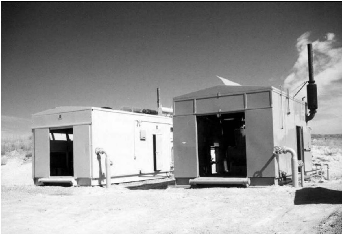
Two typical field compressors. These four-stage, 6.0 million cubic foot per day, reciprocal compressors operate at 380 horsepower and use natural gas as a fuel.
