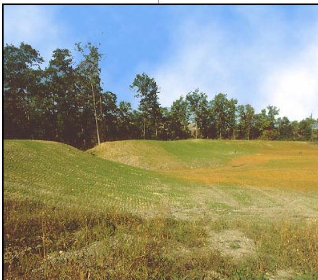
Reclamation of a sediment pond is begun when the mine site is revegetated and the need to control water runoff is no longer required.
