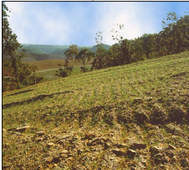
Bulldozer tracks across the slope provide niches that trap runoff for use by grass seedlings.
