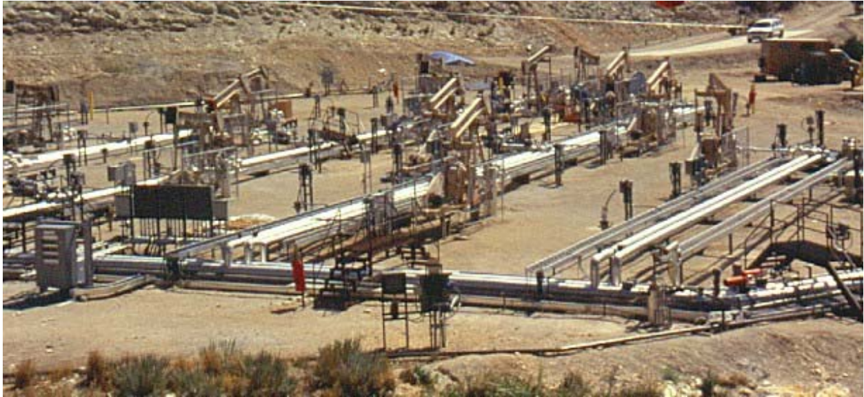
Figure 4.5 Photograph of Field Piping Network
