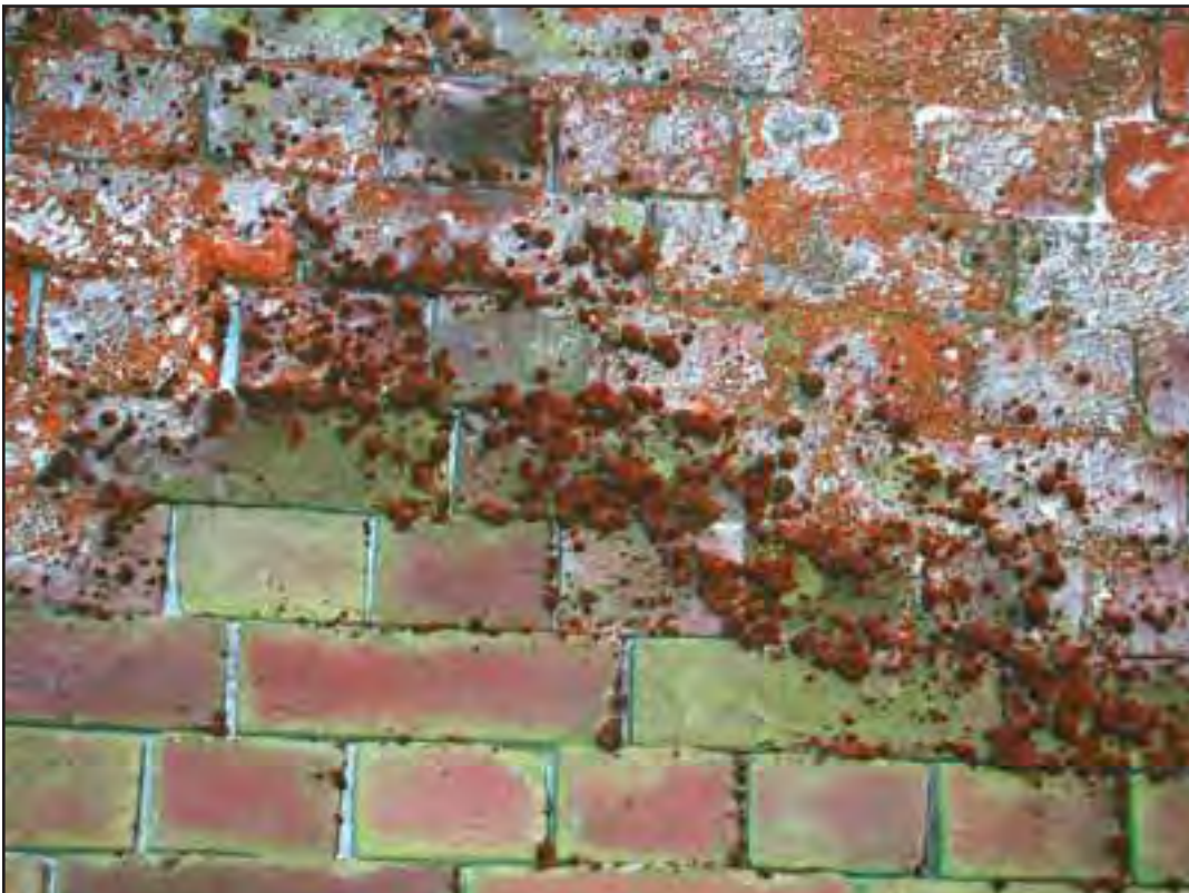
Condition Photo 4: Casemate 100; Biological growth and salts on masonry surface. (Courtesy of ARG, 2003)
