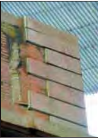
Lateral displacement is evident in the south flank parapet. (Jane Lehman, 2005)
