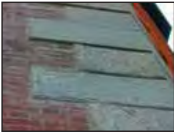
The quoins in the path of the wind and saltwater spray have lost their smooth quarried finish. (Jane Lehman, 2005)
