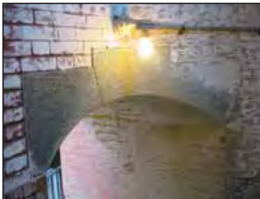
Stair #3 - The header over the openings on the 3rd tier consist of a 3-part segmental granite arch. (Jane Lehman, 2005)
