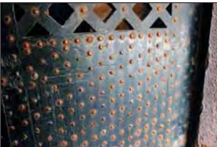
The rivets on the original wood doors rust quickly in the marine environment. (John Martini, 2005)
