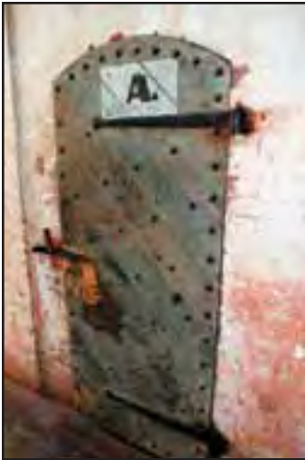
The door into jail cell 1 is original to the fort's construction. (John Martini, 2005)
