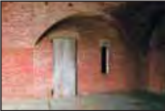
This wall was added to convert three 3rd tier casemates into a jail cell. (John Martini, 2005)
