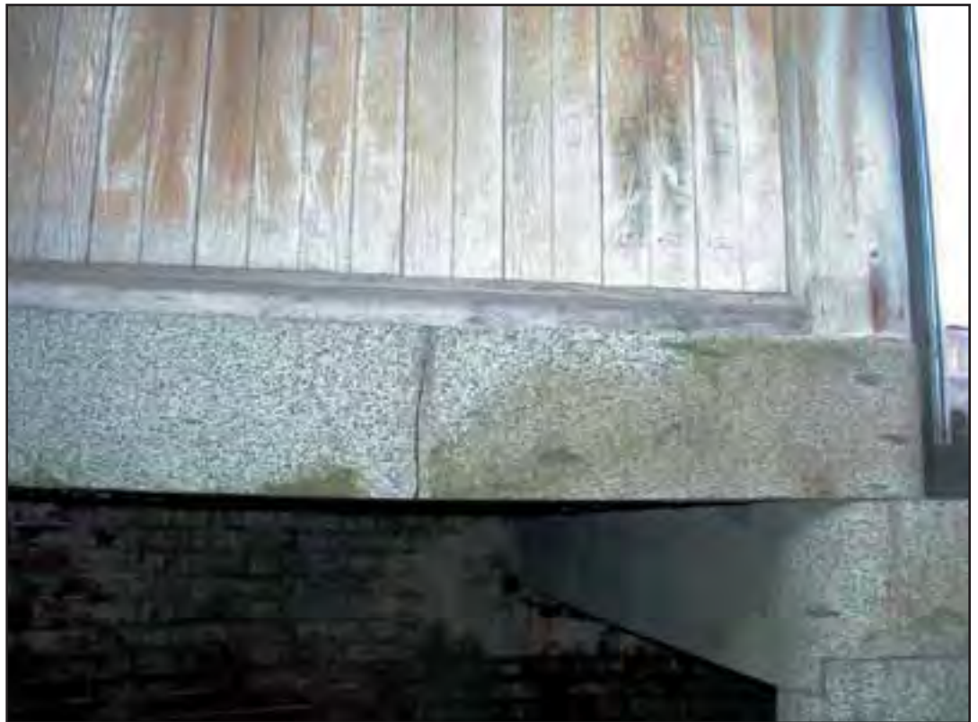
Condition Photo 6: Top Landing at Barbette Tier; Crack in granite. (Courtesy of ARG, 2003)
