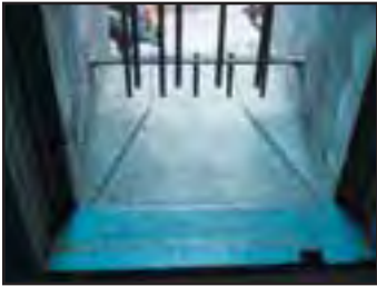
The outline of the former rifle slit is visible in all the window sills along the southwest gorge elevation. (Jane Lehman, 2005)
