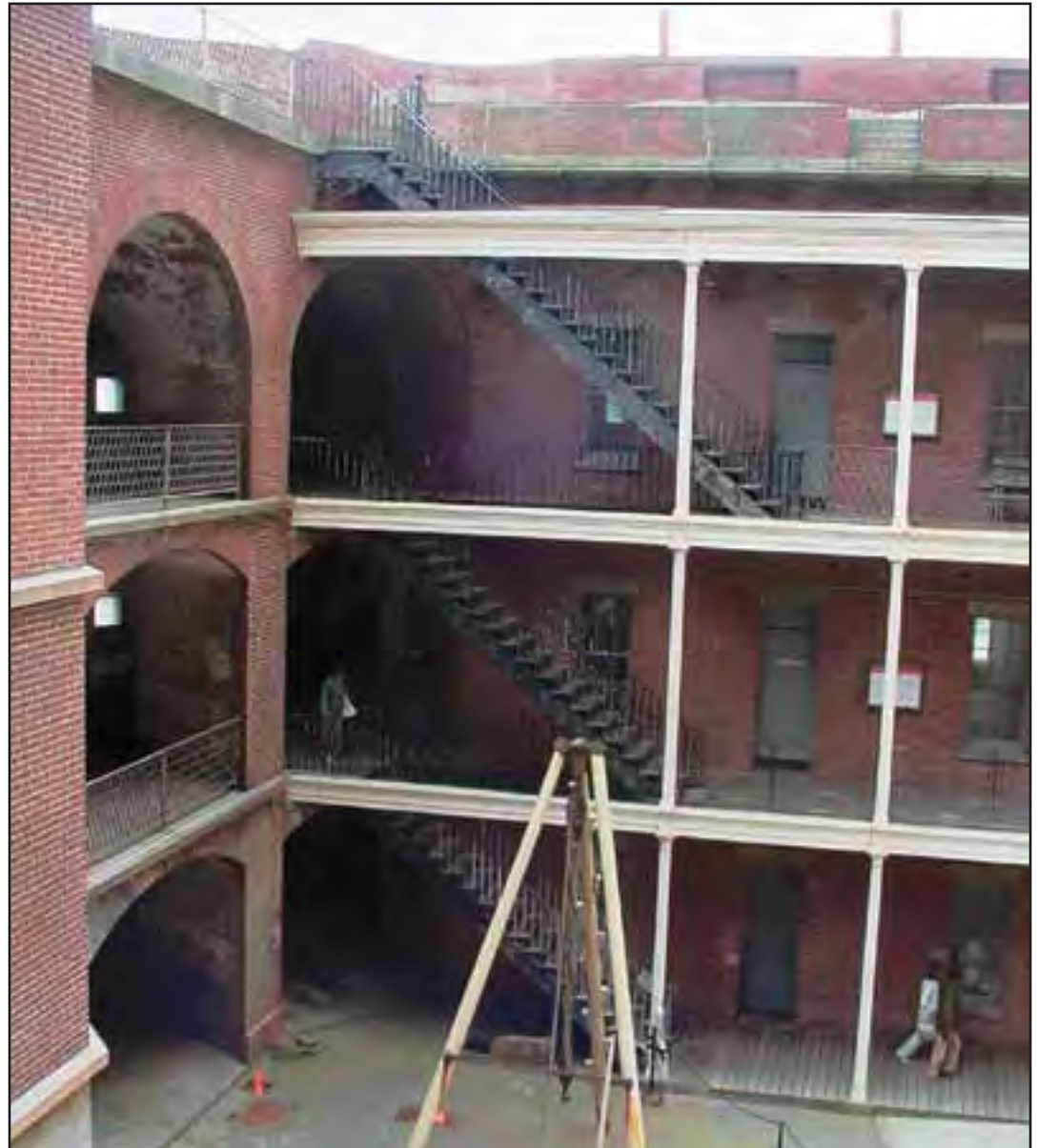
The cast iron staircase at the east end of the gallery is the only straight-run staircase in the fort. (Jane Lehman, 2005)
