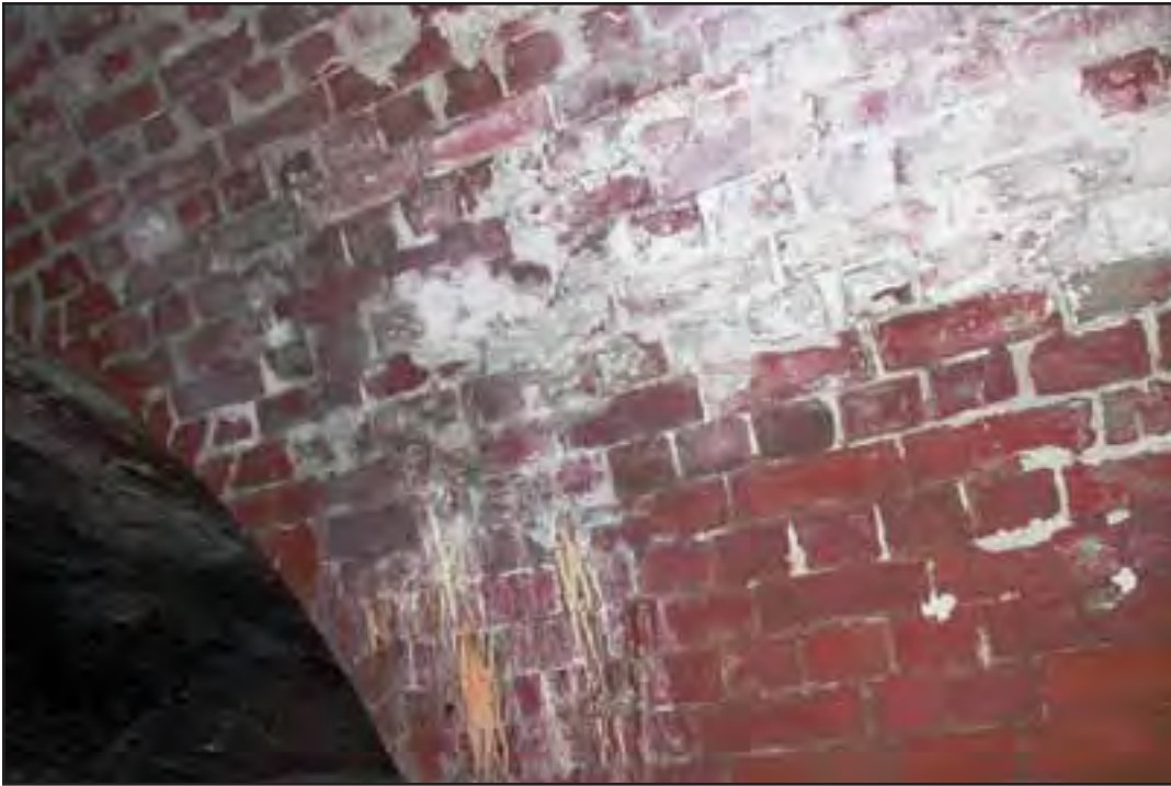
Condition Photo 3: Casemate 101; Calcium deposits are draining from open joints and coating is no longer extant. (Courtesy of ARG, 2003)
