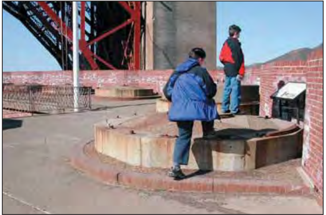
Condition Photo 5: Gun Emplacement 97; Efflorescence occurring on the brick parapet wall surface. (Courtesy of ARG, 2003)
