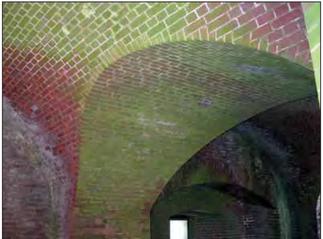
Condition Photo 2: Intersecting Arch of Casements 98 and 99; Biological growth and efflorescence settle on masonry surfaces. (Courtesy of ARG, 2003)
