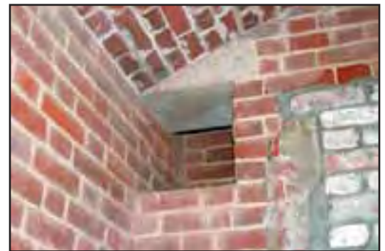
One of the square vents in the corner of each magazine with a small granite header. (John Martini, 2005)
