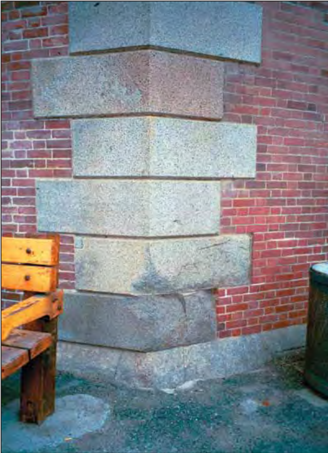
Condition Photo 7: East Bastion—East Flank; Impact damage at granite quoins and base. (Courtesy of ARG, 2003)
