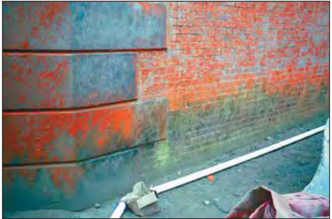
Condition Photo 1: Northwest Face Elevation; Biological growth located on brick wall and granite quoin surfaces. Exfoliation on granite quoin is due to the growth. (Courtesy of ARG, 2003)
