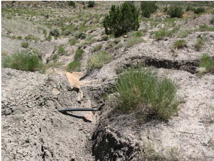
Figure 3-8: Headcutting and Gully Erosion in Drainage Areas—Existing 8-Inch Pipeline
