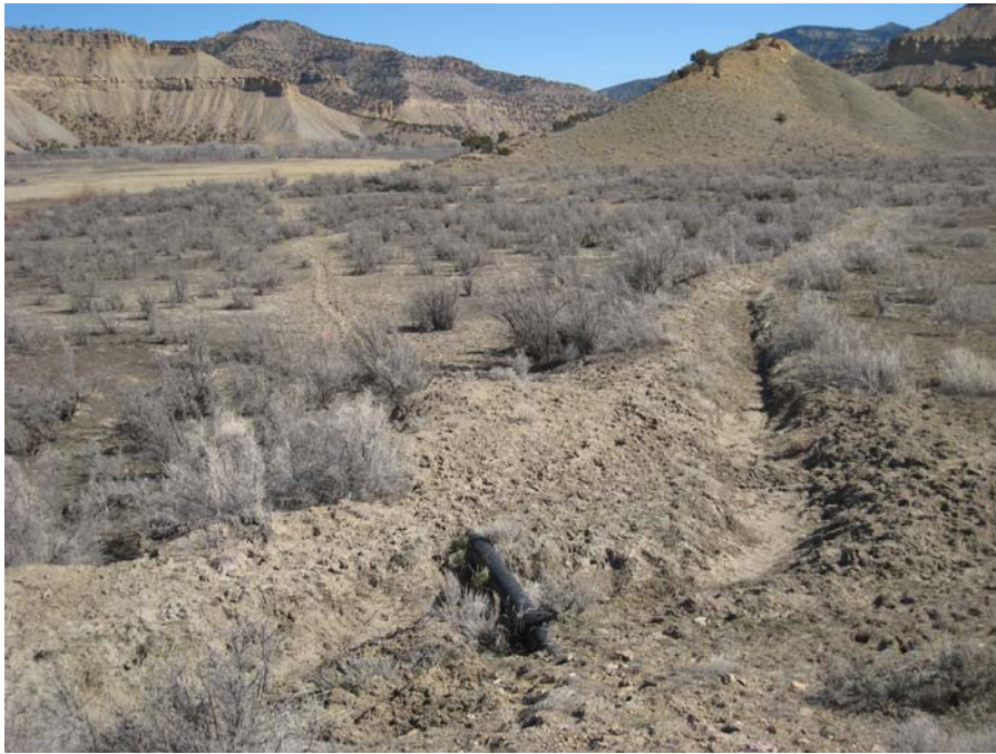
Figure 3-7: Exposure of the Existing 8-Inch Pipeline from Water Erosion
