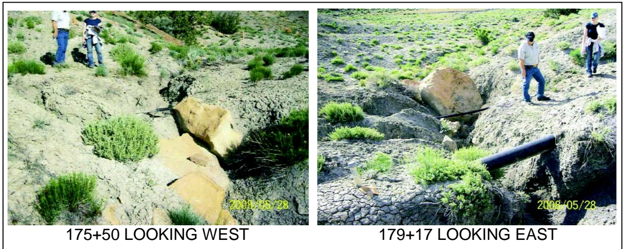
FIGURE 16 – Exposed 8" Pipe South of Mesa
