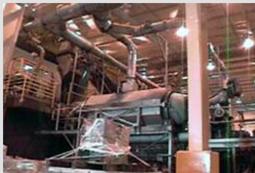
Fig. 3. Enclosed and exhaust ventilated tumbler and duct work
