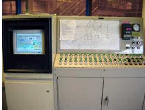
Process control system
