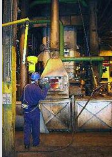
Slag tap with enclosure hooding and local exhaust ventilation
