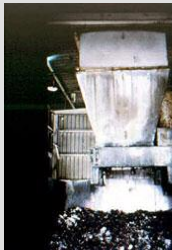
Fig.1. Enclosed and exhaust ventilated hammermill
