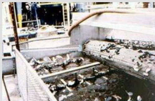
Fig. 5. Screw conveyors removing lead bearing material from a tank in the sink/float process
