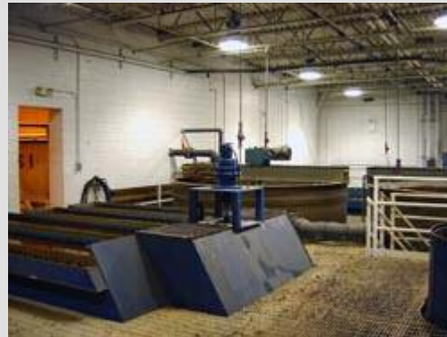
Fig. 1. Waste water treatment area
