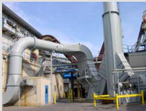
Fig. 1. Dust collection system
