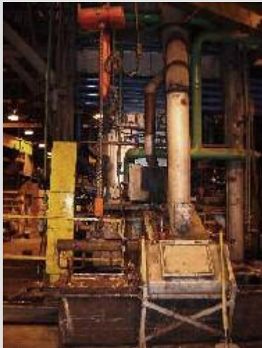
Local exhaust ventilation at lead tap
