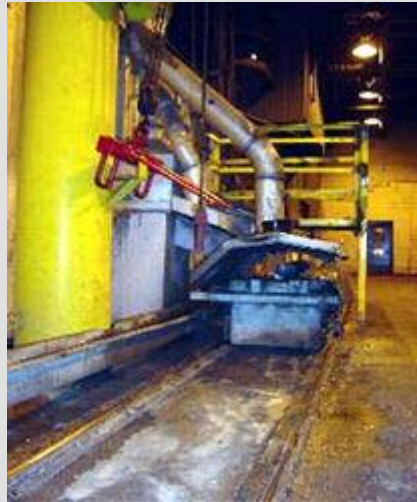
Reverberatory furnace lead tap with local exhaust ventilation
