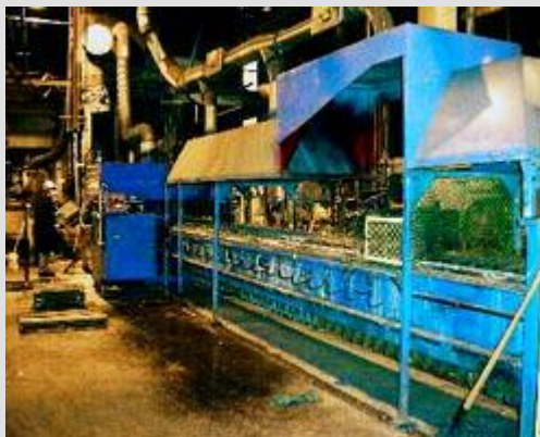
Fig. 3. Automatic casting machine with local exhaust ventilation
