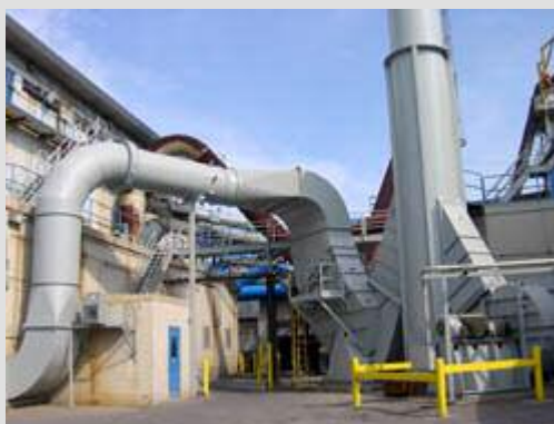
Fig. 1. Dust collection system
