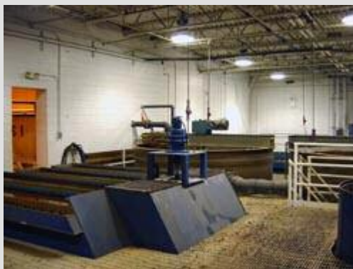
Fig. 1. Waste water treatment area
