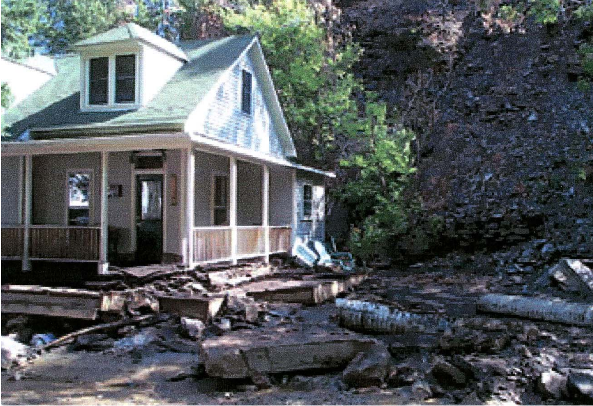
Figure 5. Photograph of erosion in Deadwood, South Dakota, following the Grizzly Gulch forest fire of July, 2002.
