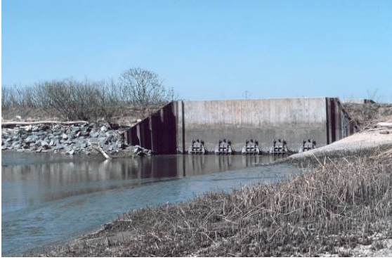
Figure 6.5: The tide gate at the mouth of Army Creek on the Delaware side of the Delaware River. The tide gate drains flood and rain water out of the creek to prevent flooding. The five circular mechanisms on the gate open and close to control water flow (courtesy NOAA Photo Library).
