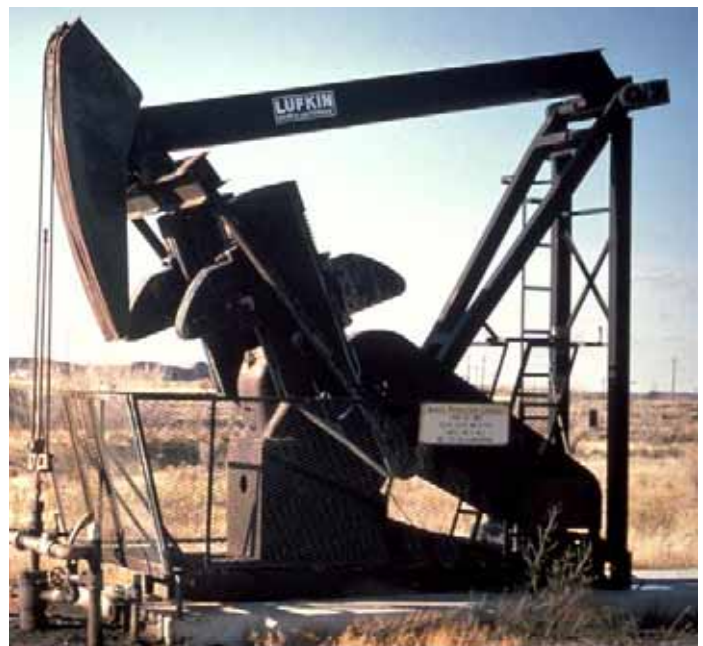
Pump that jack: Making public lands available for oil and gas leasing is an important priority for the Hollister and Caliente RMPs.
