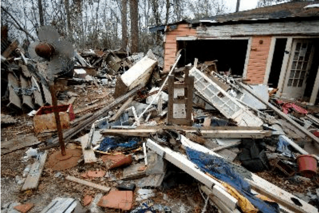
Figure 8 - Home in Waveland, Mississippi Destroyed by Hurricane Katrina
