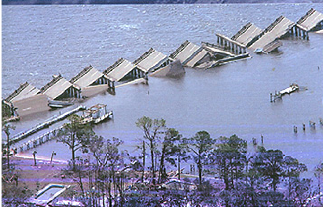
Figure 4.4 Hurricane Katrina damage to Highway 90 at Bay St. Louis, MS. (Source: NASA Remote Sensing Tutorial)
