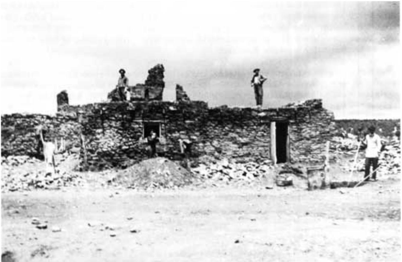
Figure 47. The Marcos Luna house at Abó. It is being converted to a toolshed by workmen under the direction of Joseph Toulouse about June 28 or 29, 1938. The Luna house can be seen in earlier photographs taken at a distance from the church, but only the lower few feet of walls still stood at the time. In 1882 Adolph Bandelier drew its outline on his map of the ruins of the pueblo of Abó, along the east edge of the mounds left by the collapse of the convento. Toulouse raised the walls by about 5 feet and added doors, windows, a roof, and a fireplace. The entire building was removed in late 1939 as part of the final cleanup of the area.
