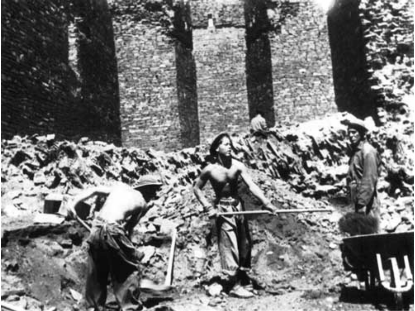
Figure 53. Removing the fill from the nave of Quarai, first week of August, 1934. The fallen east wall of the nave can be seen behind the workmen, with the stones still in approximately their original relationship to each other. The workmen are standing about on the original floor of the church.
