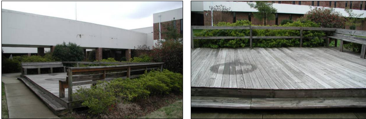
Figure 2-3. Views of ERC Deck (note that moisture stains were temporary and that boards under benches were not used to construct minidecks)
