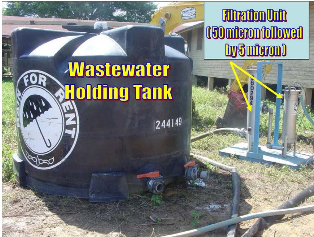
Figure 4-11. Water filtration system and holding tank.
