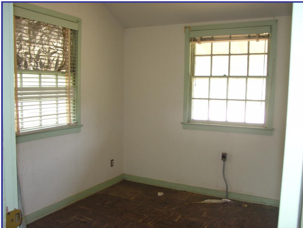
Figure 3-4. Interior view of Building #3607 (AACM). Interior finishes are gypsum wallboard (ceiling and walls) and nine-by-nine-inch resilient floor tile.
