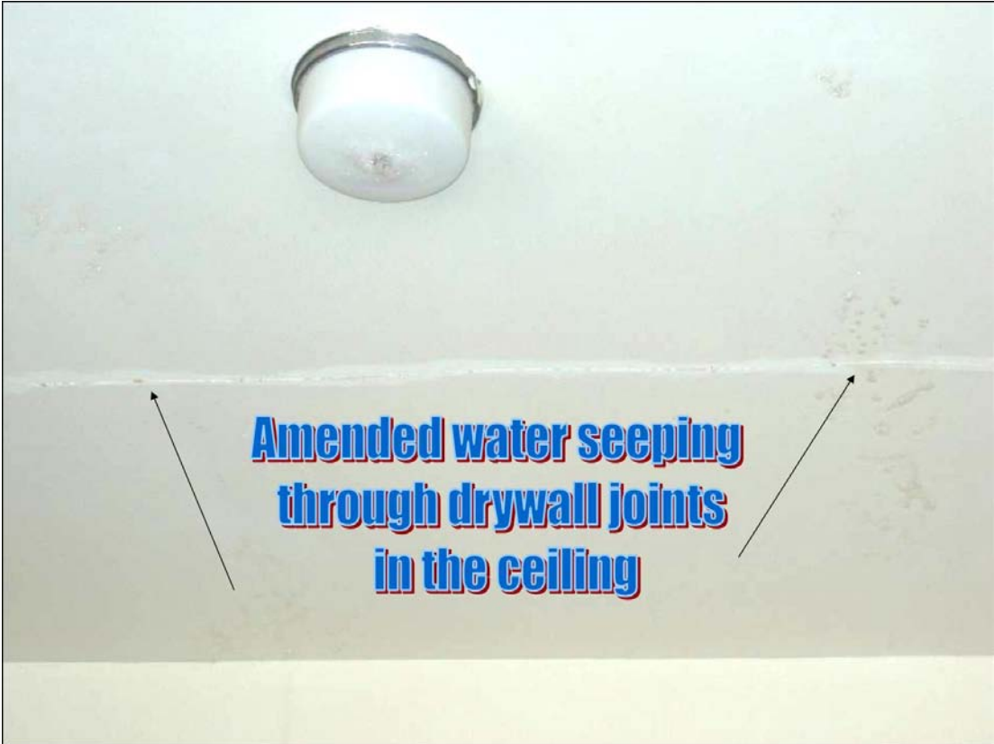
Figure 4-26. Amended Water seeping through ceiling drywall joints.
