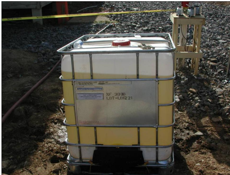
Figure 4-21. Wetting agent supply tank for the AACM demolition.
