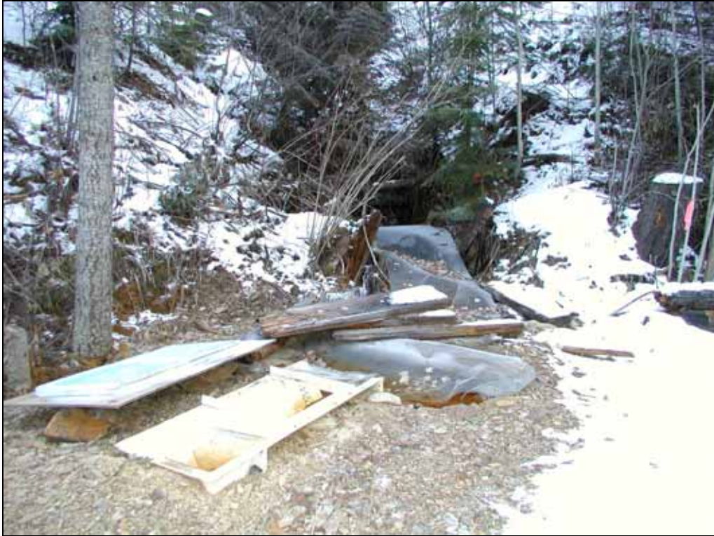
Figure 2-5. Sixty-degree trapezoidal flume used to direct NSM adit discharge through the ATS.
