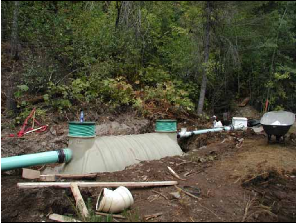
Figure 2-8. ATS Tank 1 (retention basin) used to trap debris in water.
