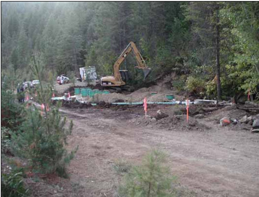
Figure 2-11. ATS system uncovered with risers and sample ports constructed.
