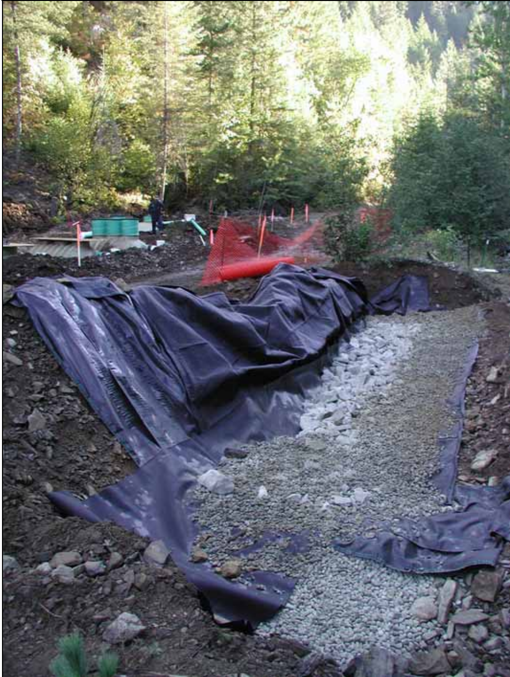
Figure 2-7. ATS catch basin for effluent water.
