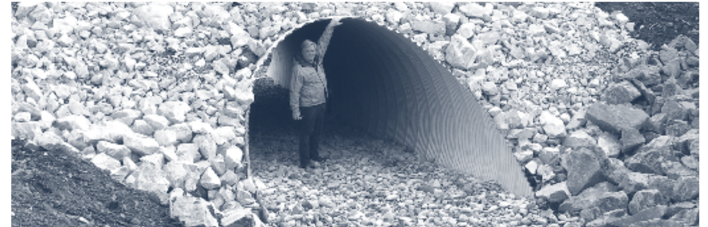
The new culvert at Beaver Creek is the same level as the natural stream channel. Gravel inside the culvert slows down the water and allows fish to swim upstream more easily. Culvert project engineer Don Porior of North Bend, Oregon, shows the size of the new culverts.
