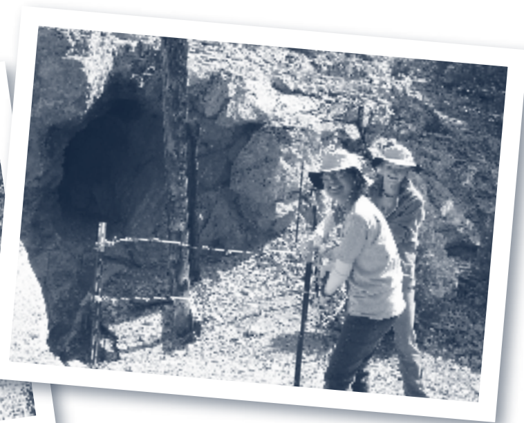
Christina Martinez (front) and Jenny Giraudo build a barbed wire fence to warn people of a dangerous mine adit.
