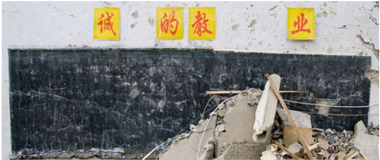
The interior of a school classroom is destroyed by an earthquake that struck Dujiangyan, Sichuan, China, in 2008.
