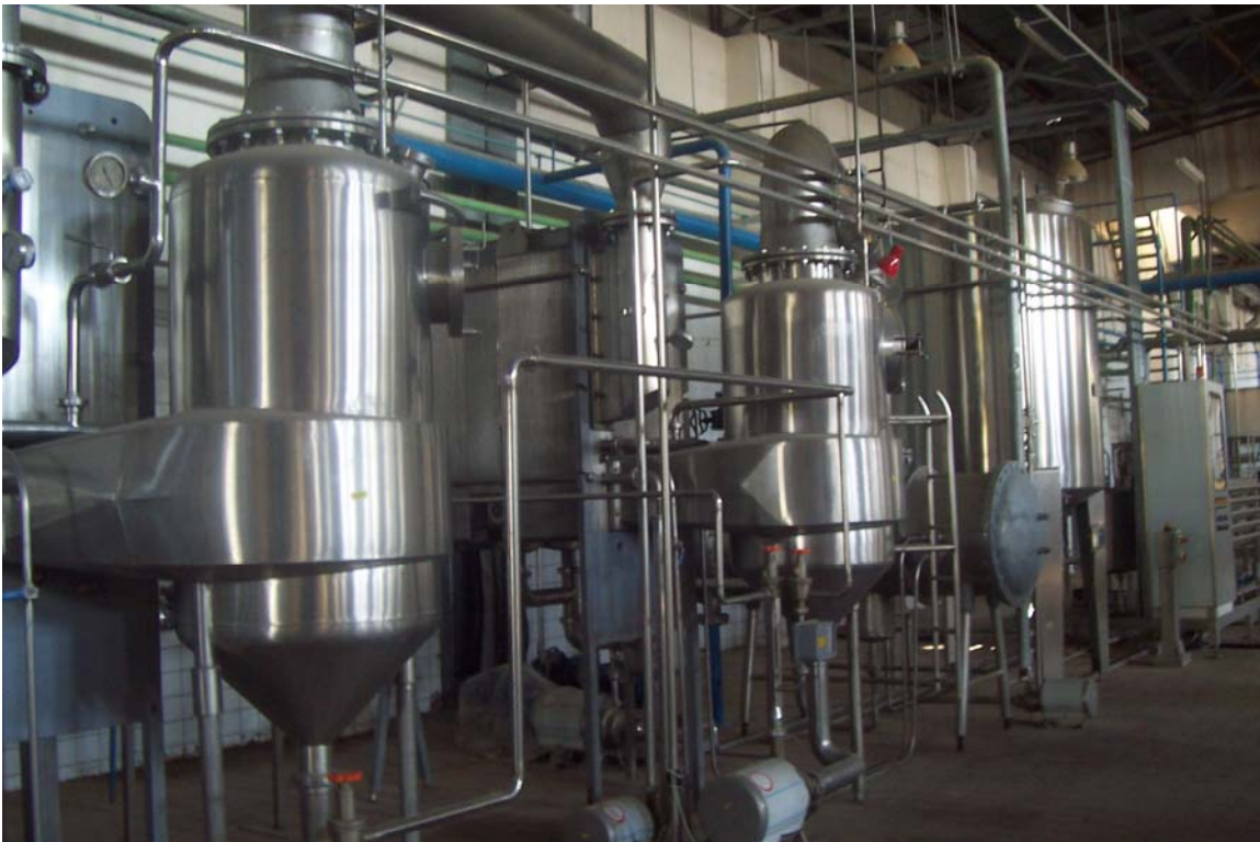
View of part of the juice line at the Harir Factory. Much of the machinery has undergone no more than ten days' operation time since installation in 2003.
