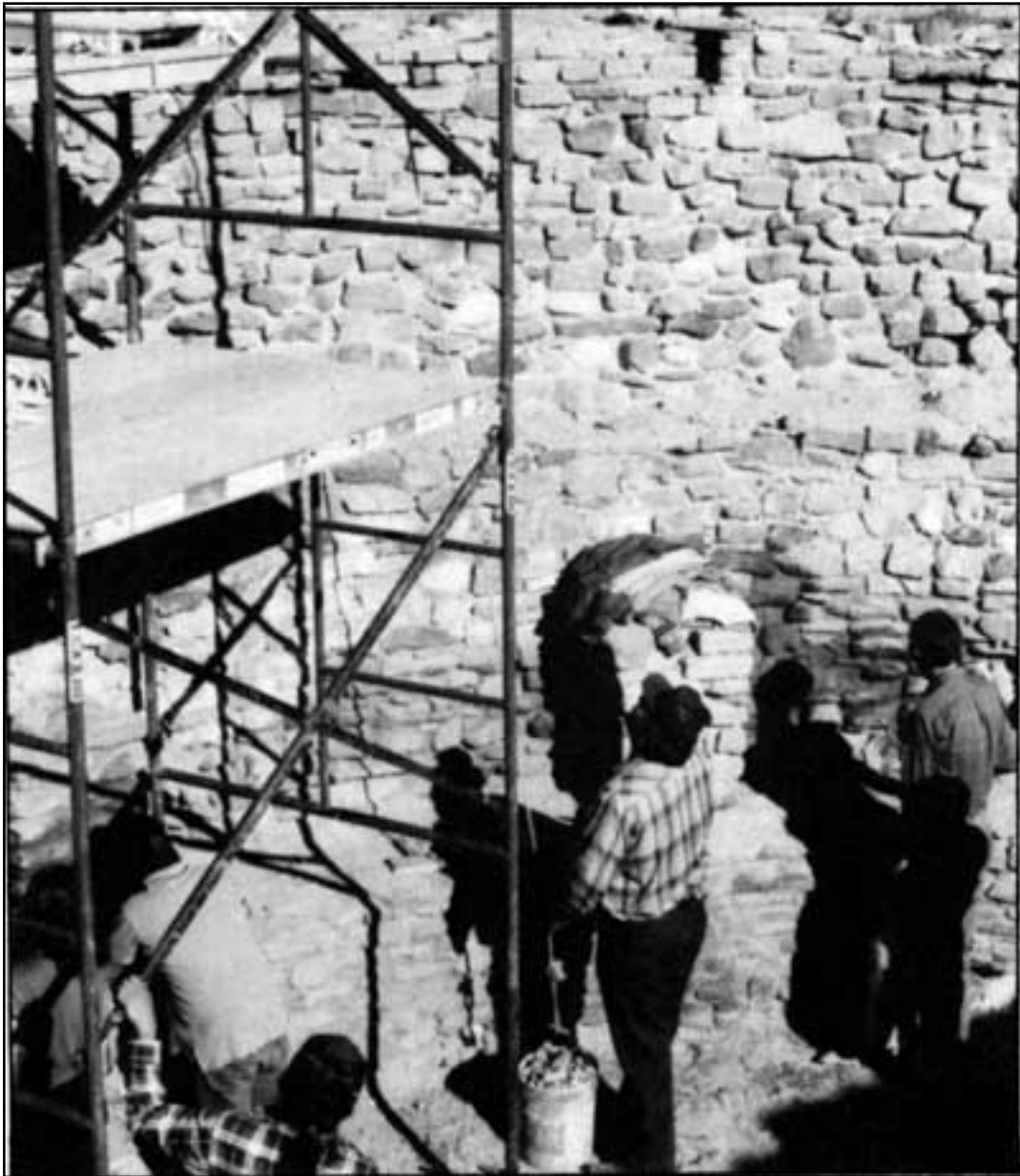
Figure 12.7. Routine maintenance stabilization at Aztec Ruins being done in connection with regional training exercises, May 1989.
