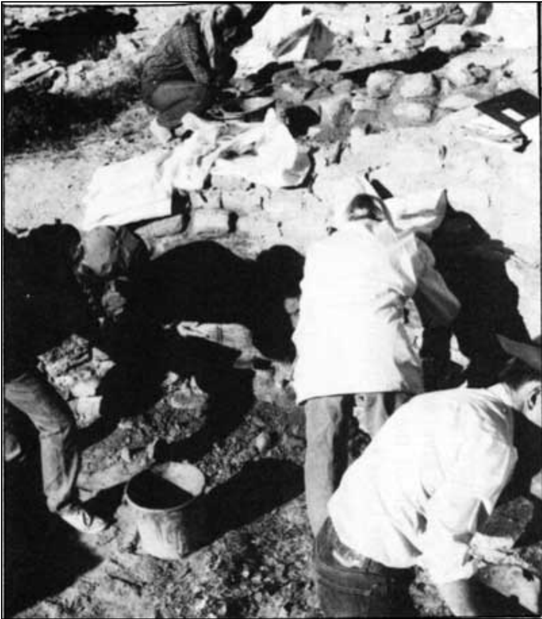
Figure 12.6. Routine maintenance stabilization at Aztec Ruins being done in connection with regional training exercises, May 1989.
