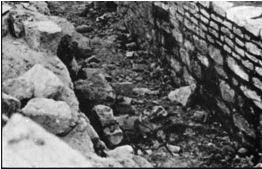
Figure 7.7. Resetting exterior wall of North Wing, 1934. Rubble core and shaped sandstone veneer evident.
