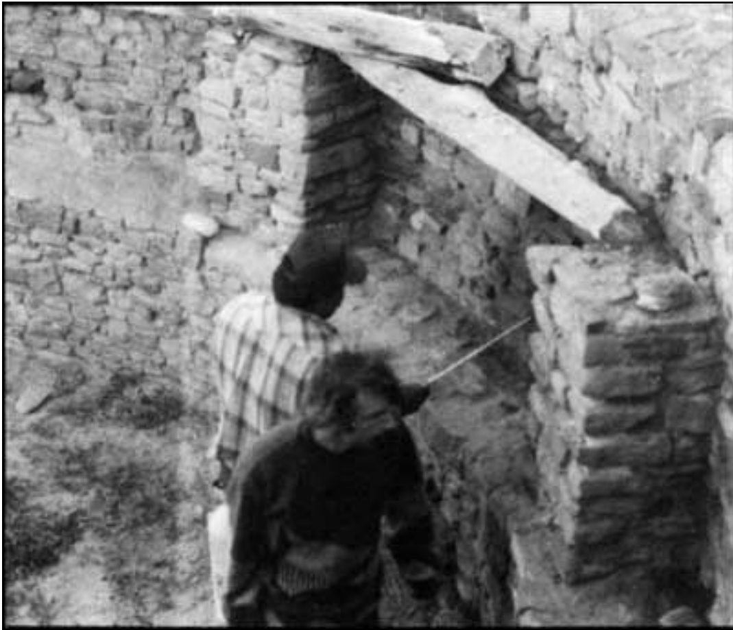
Figure 12.9. Routine maintenance stabilization at Aztec Ruins being done in connection with regional training exercises, May 1989.
