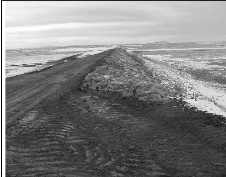
Rehabilitation of the Valley County #2 reservoir in eastern Montana included widening the embankment and installing rock riprap on the upstream face.
