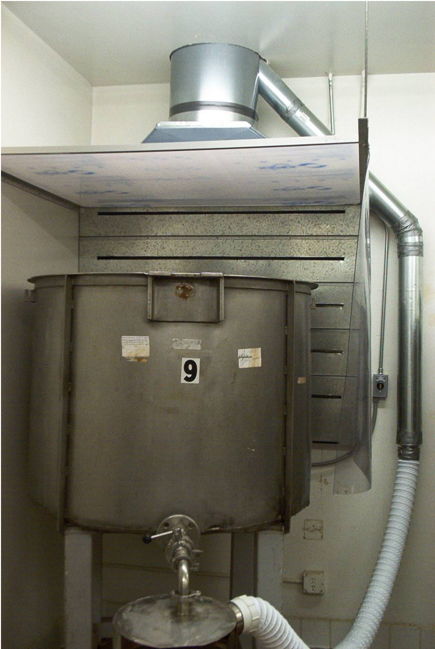
Figure 3. Ventilated booth-type exhaust hood.
