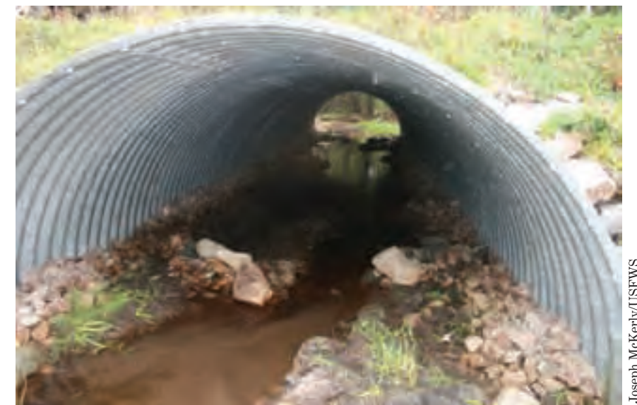
Fish habitat fills this arched culvert throughout its length, allowing Atlantic salmon, brook trout, turtles and aquatic bugs to pass under the road without hinderance.
