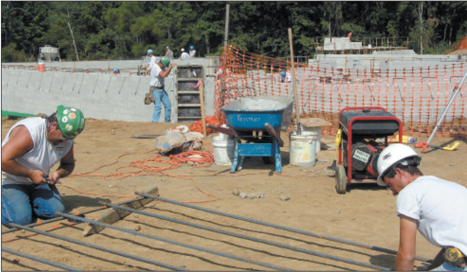
A hive of activity at the construction site for the park's new museum.
