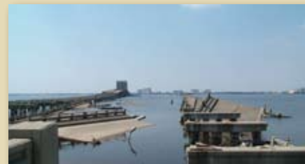
Hurricane Katrina damage to bridge
