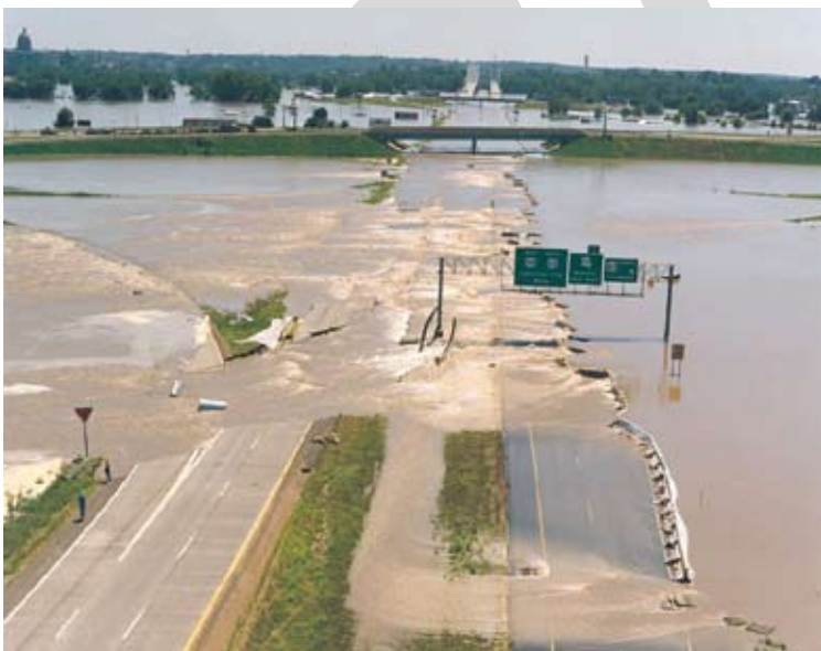
The Great Flood of 1993 caused flooding along 500 miles of the Mississippi and Missouri river systems. The photo shows its effects on U.S. Highway 54, just north of Jefferson City, Missouri.
