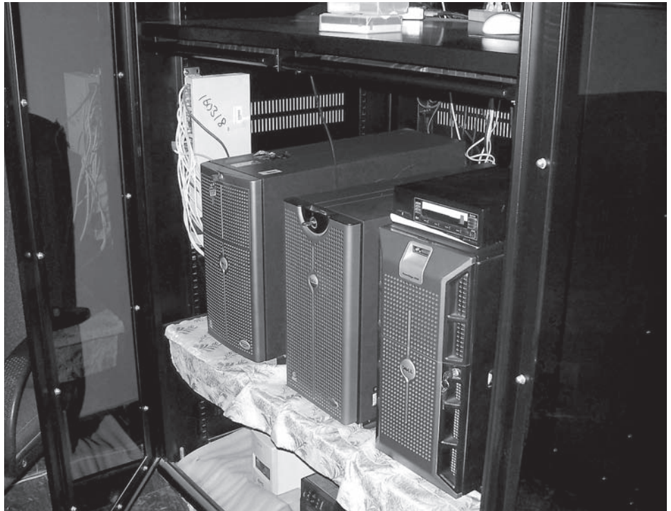
Figure 12: Servers Used to Store Identification Data at MOI Headquarters in Kabul
