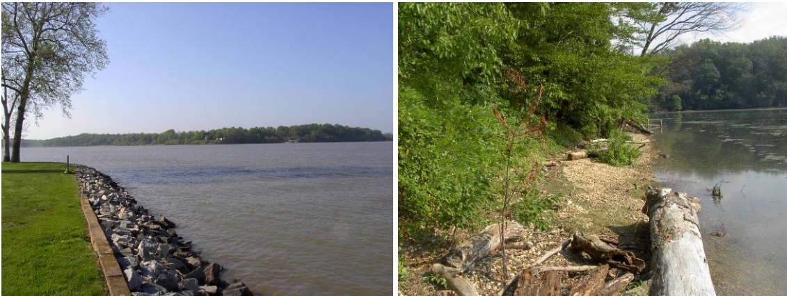
Figure 12.4 Hard and Soft Shore Protection. (a) Stone Revetment along Elk River at Port Herman, Maryland, May 2005 (b) Dynamic Revetment along Swan Creek, at Fort Washington, Maryland, September 2008.
