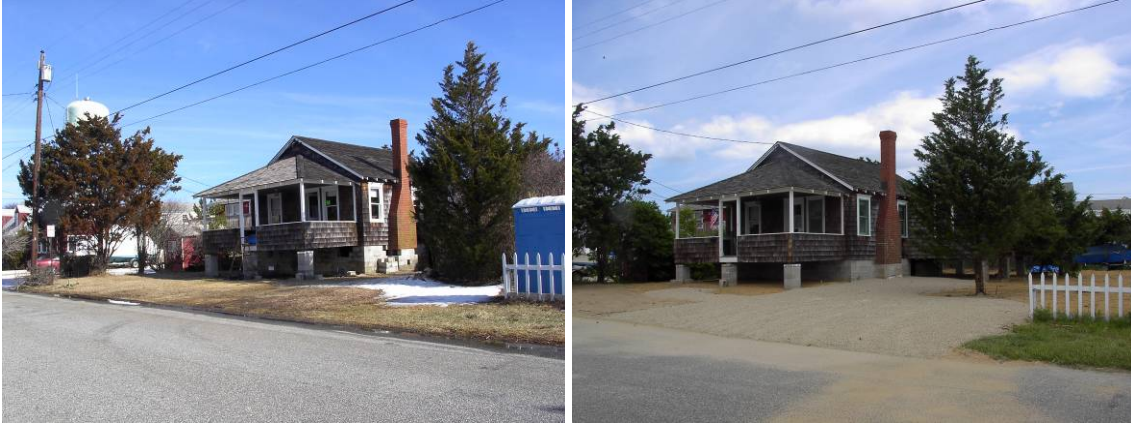
Figure 12.5 Elevating land and house. (a) Initial elevation of house in Brant Beach (New Jersey). (b) Structural beams placed under house, which is lifted approximately 1.5 meters by hydraulic jack in blue truck. (c) Three course of cinder blocks added then house set down onto the blocks. (d) Soil and gravel brought in to elevate land surface. (January through June 2005)
