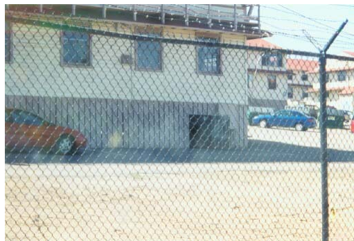
Photo 21: All of the Historic Barracks facilities are candidates for incineration by wind blown embers getting under the structures. All of these structures lie up hill from the heavily vegetated east slope. A Santa Ana driven fire with ember laden winds would destroy most of these facilities. National Historic Preservation Act Sec. 106 compliance would be required.
