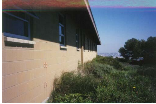
Photo 16: A close-up of the same building shown in Photo 15 with brush growing up to the structure. The radiant heat from a fire burning up slope could blow out the windows and the embers rising up the wall could ignite the overhang eave resulting in the loss of the structure.
