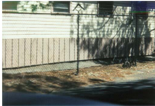
Photo 20: This skirting will still permit the passage of wind blown embers. Also note the pine needle litter next to the structure. This structure lacks survivable space which would be very easy to achieve.
