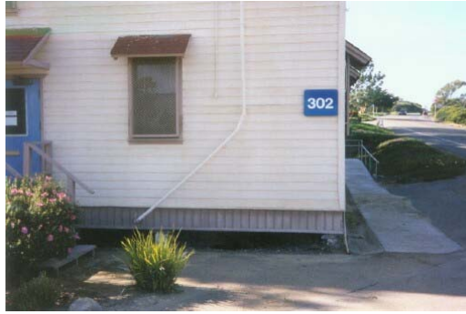
Photo 19: Many of the military buildings on Point Loma were set up as temporary structures. They were built on piers with no foundation. Wind blown embers can lodge beneath these structures resulting in their incineration. This building is northwest of the Fire Station (photo 17). Solid skirting should be installed on all of these structures. National Historic Preservation Act Sec. 106 compliance would be required.
