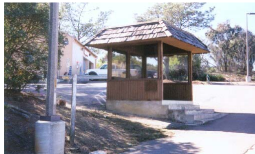
Photo 18: The combustible wood roof on the bus stop in front of the Fire Station should be replaced with a non-combustible roof covering. In a wind driven wildfire the shingles will readily ignite and blow off as flaming firebrands that will ignite combustible material and start new spot fires.
