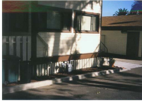
Photo 25: All of these beautiful homes are built on pilings. The current skirting will allow the passage of wind blown embers from the eucalyptus trees to blow beneath the buildings, potentially causing the loss of the structure. A solid skirting would prevent such a possibility. National Historic Preservation Act Sec.106 compliance would be required.
