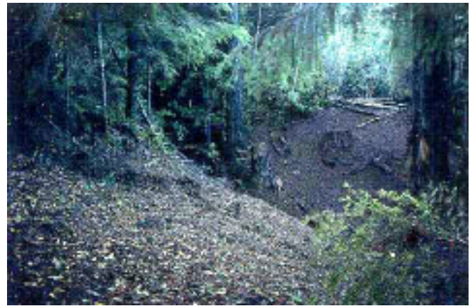
After restoration: The road bench is obliterated and the hillslope is recontoured to mimic the natural hillslope uncovered during excavation. Exhumed stumps indicate the location and elevation of the original hillslopes. Photo: NPS
