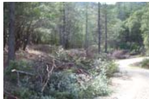
Crews spent the summer cutting, stacking and chipping brush 50 to 100 feet on both sides of the road.
