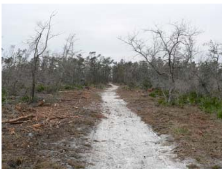
Before (Top), Posi-Trac Clearing Fuel Break (Middle), and After (Bottom) Mechanical Fuels Reduction
