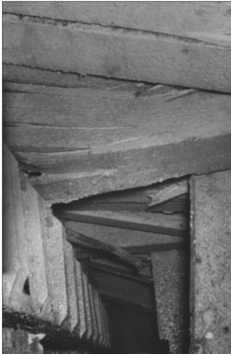
View looking down a manway after a burst crushed it. The normal condition of the manway would be a four foot square smooth sided opening. Photo courtesy of ASARCO taken in the Galena Mine in the Silver Valley.
