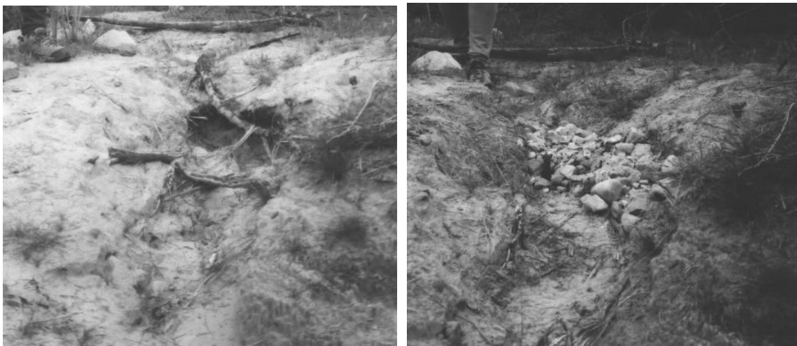
(A) Knickpoint advancement at C:13:100 and a knickpoint treatment constructed in FY2005.
