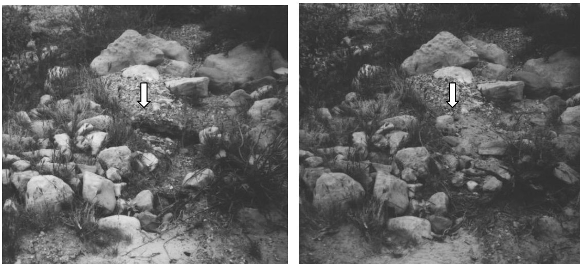
(B) Headward advancement at C:13:099 and a headcut treatment constructing in FY2005.
