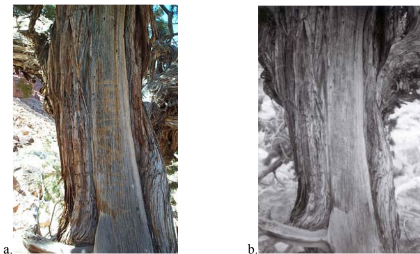
Figure 12. Graffiti recorded by NPS archaeologists at site C:05:007 in May 2002 (Photo a). On 3-18-03 base Park archaeologists (Jan Balsom and Grace Ellis) removed the graffiti with sandpaper (Photo b).
