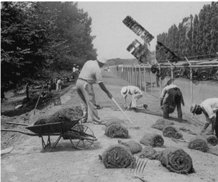
Figure 23 - Laying sod on flood levee to stabilize the earthen berm, August 4, 1936. MRC 2-127.
