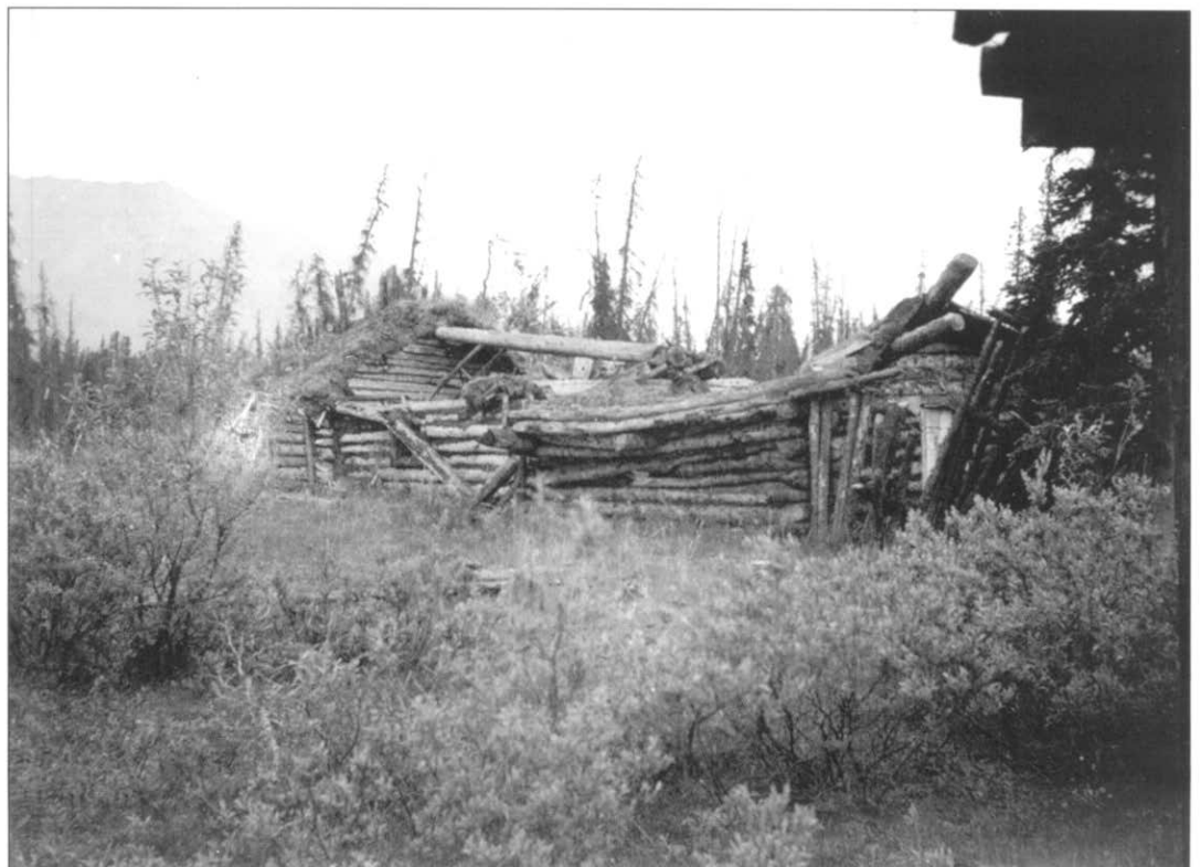
When Superintendent Frank Been visited the Sheldon Cabin in June 1941, the 34-year-old original cabin and the 1914 addition were both badly deteriorated. DENA 4-5, Denali National Park and Preserve Museum Collection
