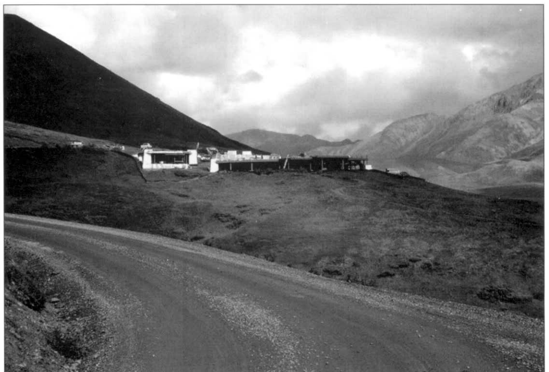
The new Eielson Visitor Center, seen here under construction in 2006, opened in the early summer of 2008. NPS Photo
