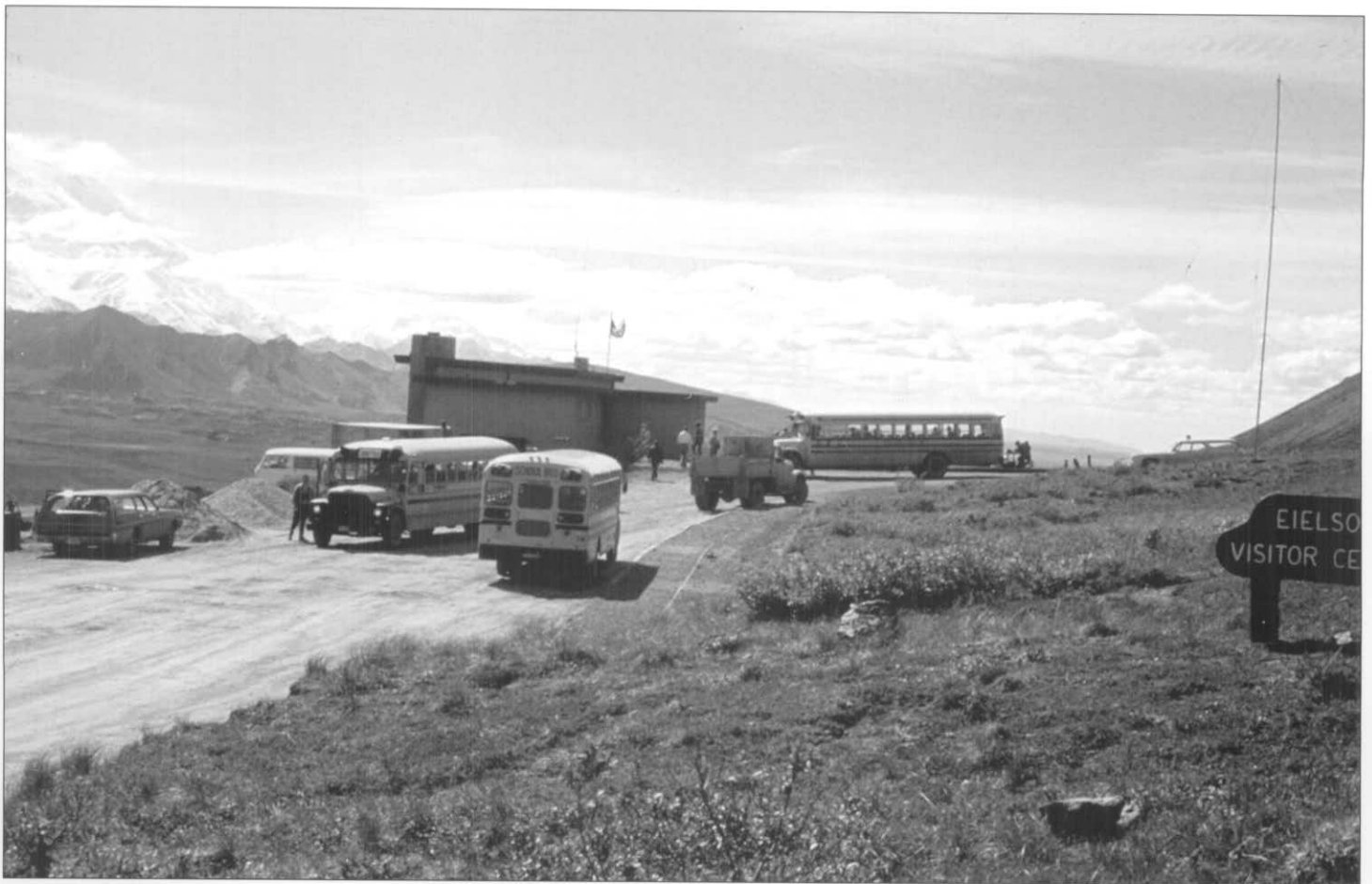
By July 1974, construction of additional restroom facilities, a new entryway, covered walkways, and an open observation tower were underway at Eielson Visitor Center. DENA 5749, Denali National Park and Preserve Museum Collection
