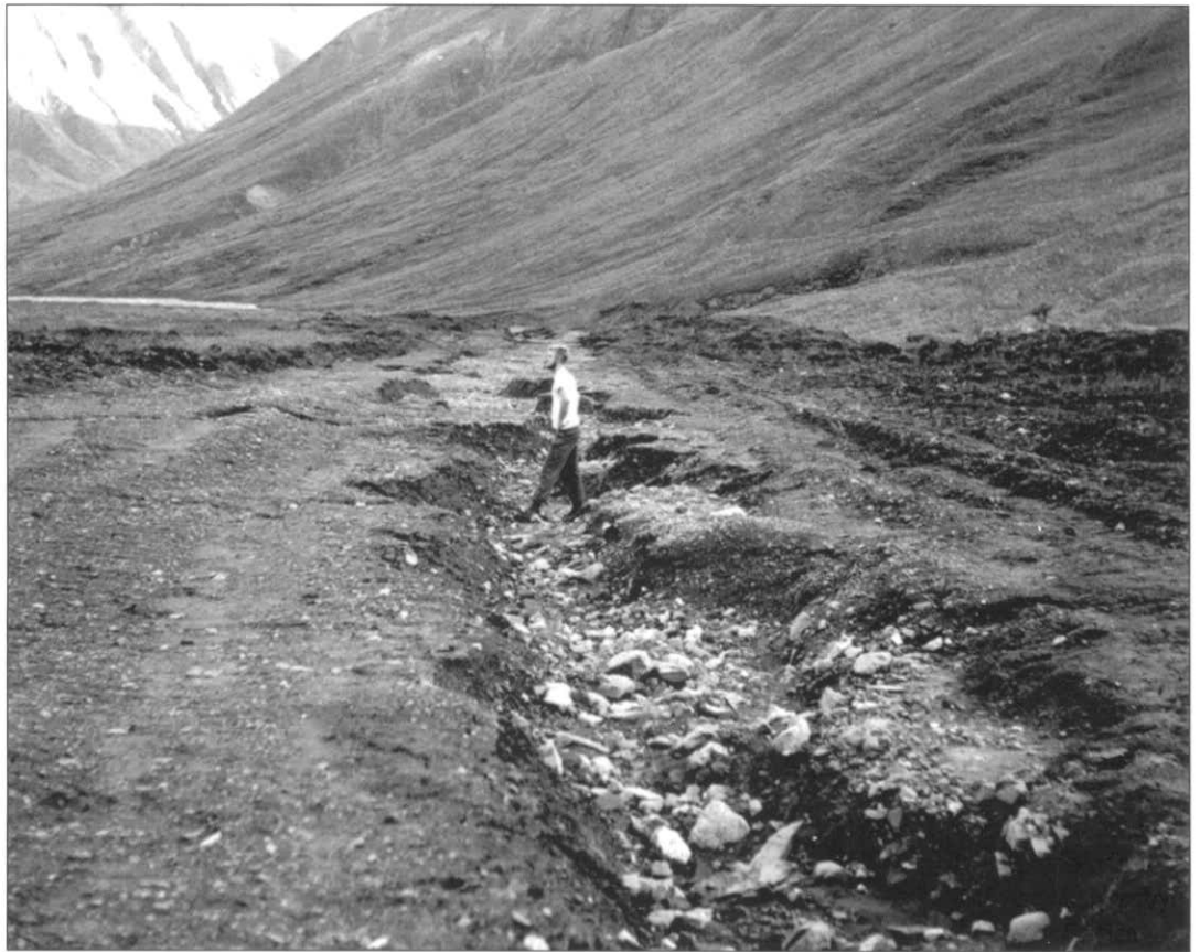
By September 1963, when this photo was taken, the 7-year-old landing strip on the West Fork of Windy Creek (which was adjacent to a potential limestone development area) had suffered considerable erosion. DENA 16-33, Denali National Park and Preserve Museum Collection
