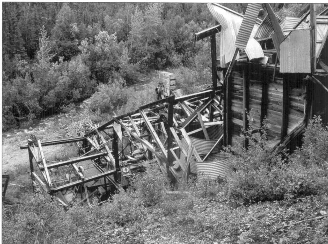
What remains of the Stampede Mine mill structure is shown here in 2003, looking down on the ruins and Stampede Creek below the mill. NPS Photo
