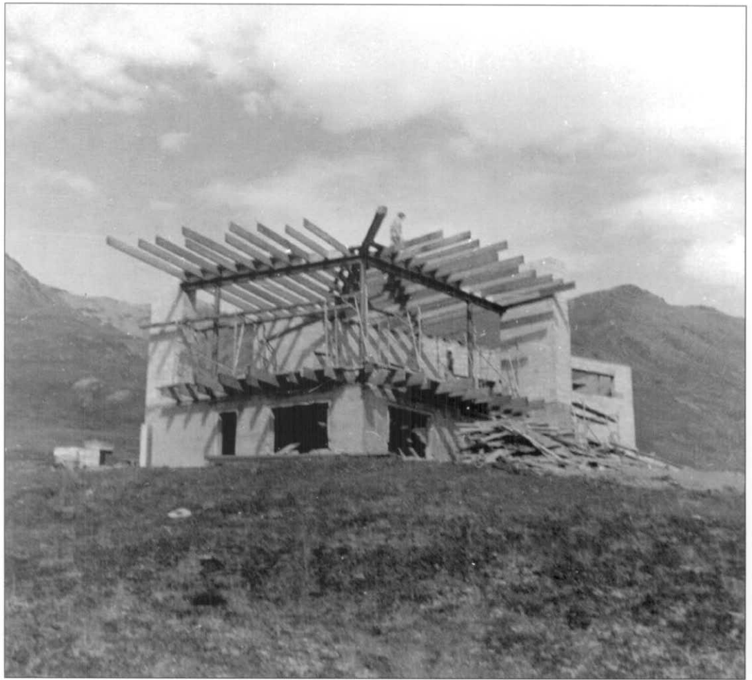
Construction of the Eielson Visitor Center was well under way in this September 1959 photograph. This Mission 66 visitor center opened to the public in July 1960. DENA 5-8, Denali National Park and Preserve Museum Collection
