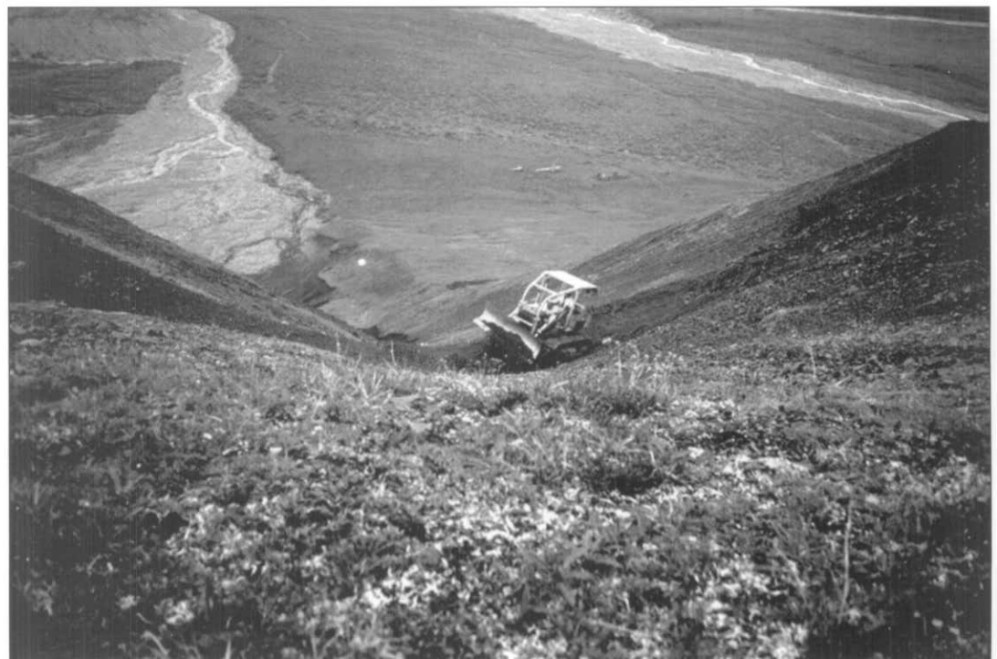
The bulldozer that was brought to Slippery Creek by the mine operators in 1969 was used during reclamation of the mine road on Mineral Mountain in 1987. The Slippery Creek cabin can be seen at the base of the mountain. Brad Ebel Collection
