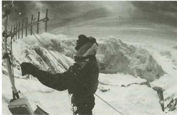
NPS Photo Rangers installed a new weather station at the 14,200 foot level on McKinley this past year.
