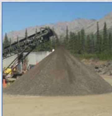
We remove cracked and rutted asphalt and crush it for later reuse. In 2005, 700 cubic yards of asphalt were recycled.
