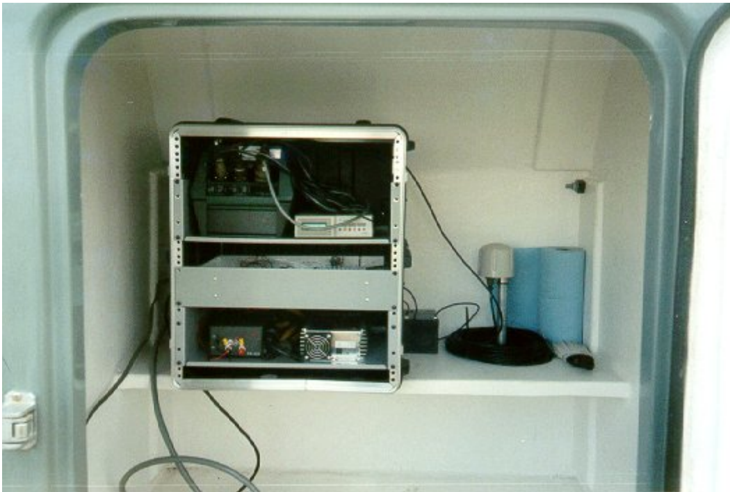
Figure 2.3. Inside of typical hut where instruments are housed. Huts are locked or bolted closed to prevent animals from intruding.
