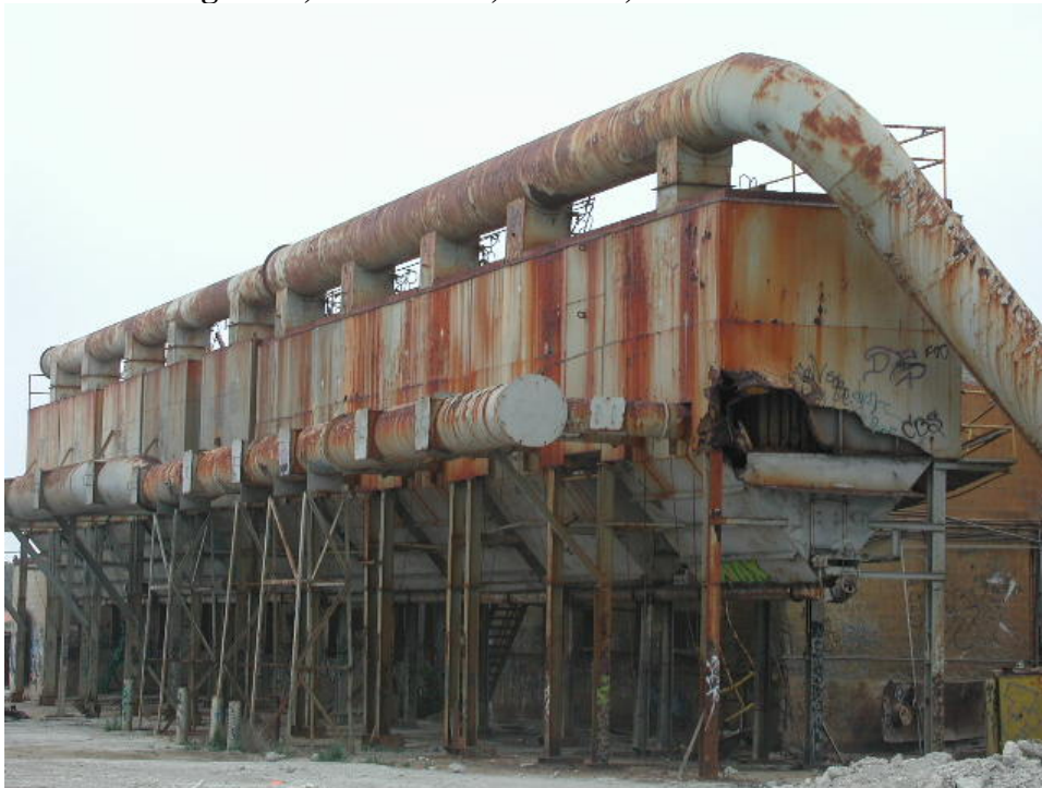
Photo taken during staff visit of Halaco site, June 2007.
