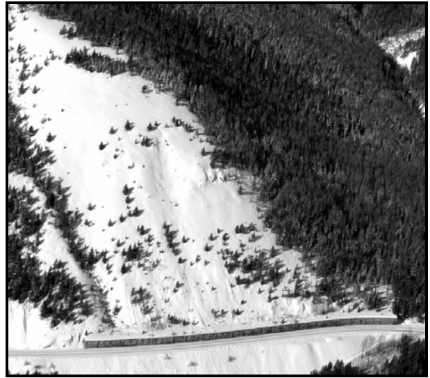
Figure 6: Aerial photo of burned-out snow shed (4-C) showing steep, unconfined avalanche path. Photo by D. Stoneman.
