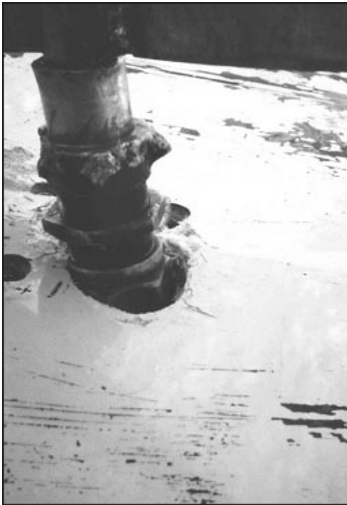
Photo 1: A Failed Rudder Post Housing
